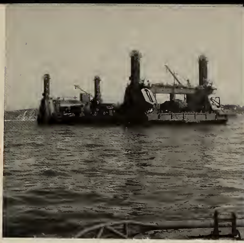
6. The wharf for unloading the ships inside the breakwater was made of floating pierheads. Above, one of them is seen waiting to be towed into position. The pillars at the corners are adjustable legs, lowered according to the depth of the water, to anchor the pierhead to the sea bed.
